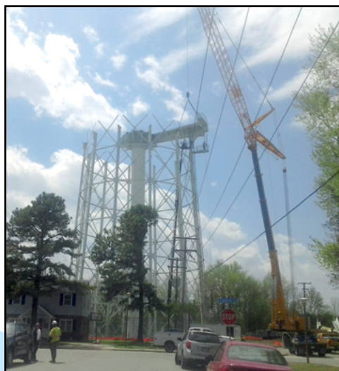
Travelers crossing the Hampton Roads Bridge Tunnel will no longer be welcomed to the Peninsula by the Phoebus water tank, which was taken down in March and April.
